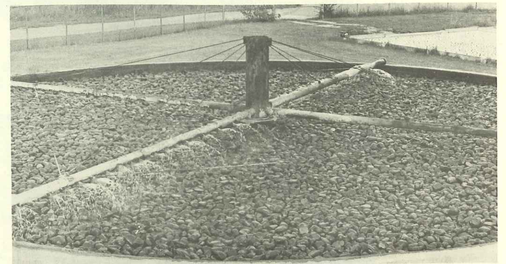
Trickling Filter System
